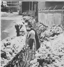
WORKMEN LAY reinforcing steel in a ditch near No. 1 Powerhouse for transformer cable conduits, then fill the ditch with cement. Top photos show general views of the transformer installation.
